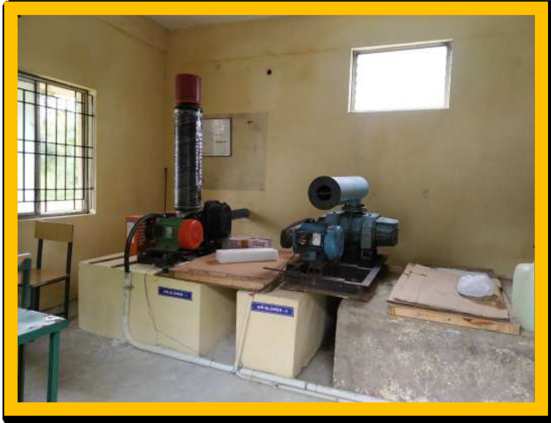
STP AIR BLOWER
